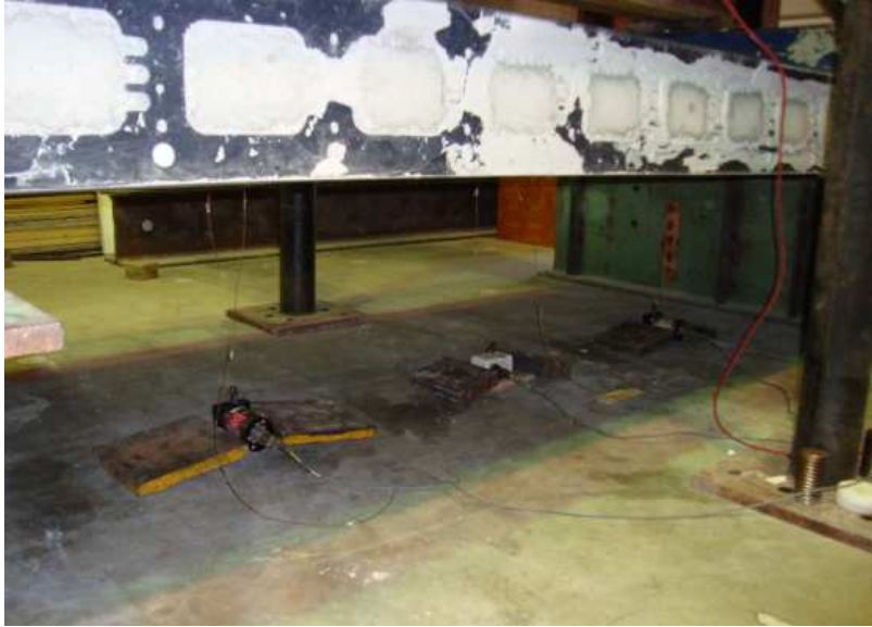
Figure 14. Displacement Transducer Placement
